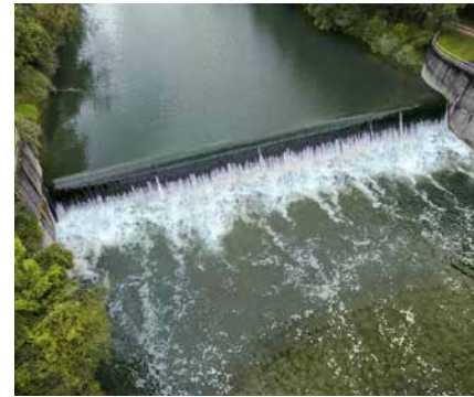
The Arlach weir and the Heimertingen sill are to be converted into a more natural condition.
