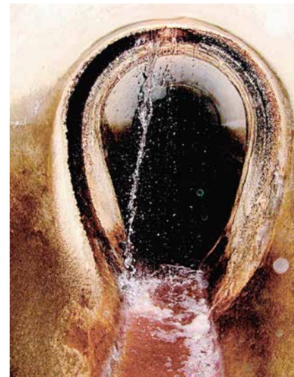
Sewer system damage: a sewer pipe wall is severely damaged by a supply pipeline (upper photo) crossing directly through it; groundwater ingress due to a leaky sewer (lower photo).
