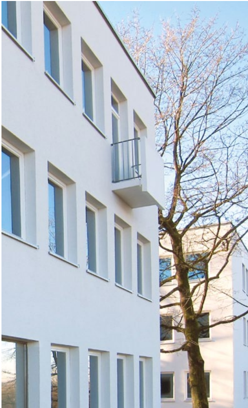
Technische Universität München (TUM) Freising-Weihenstephan: Energy-efficiency refit as part of the special programme
