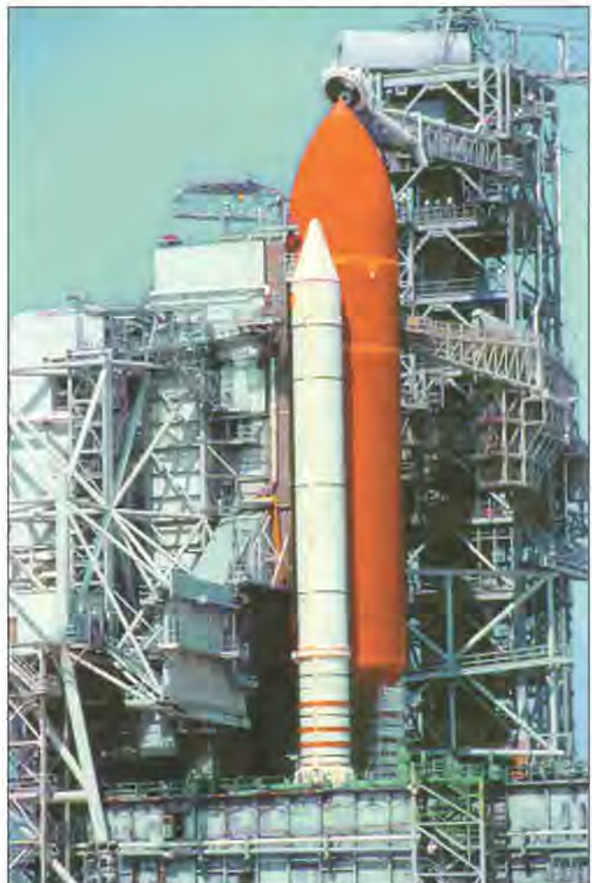
Fig. 1. The Space Shuttle Discovery on its launch pad following repair of 208 holes that had been made in the insulation by a Northern Flicker. The repaired holes can be seen as light spots in the rust colored insulation.
