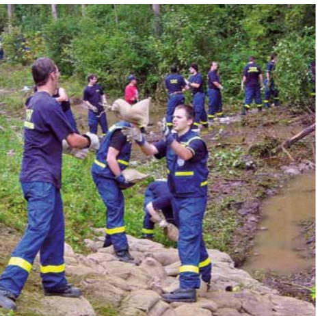
Floods in August 2005: Emergency task forces securing a dyke structure – in this case the disaster relief organisation Technisches Hilfswerk
