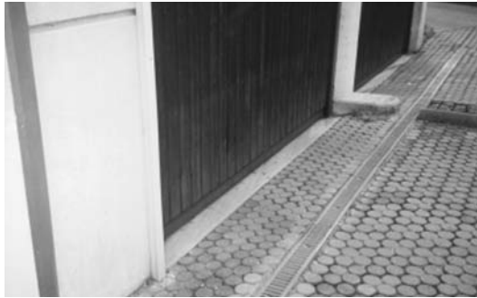
Fig. 23: Example of a drain resp. rain gutter near an enclosed underground car park entrance
