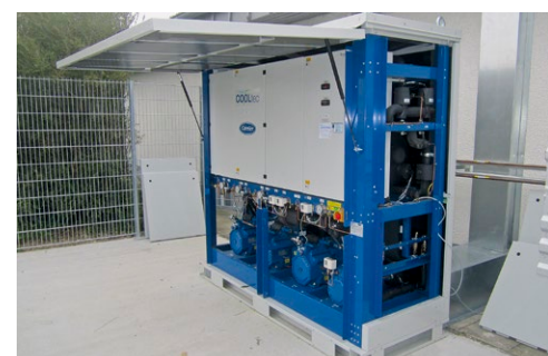
Left: A sketch of the CO 2 Plant Below middle: The central control cabinet Below right: The control cabinet and the compressors are placed in a compact box outside of the supermarket
