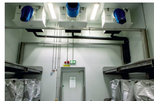
Right below: the direct expansion diffusers of the CO 2 plant for cooling the room and the smaller propane modules of the refrigeration system Left below: Sketch of the cooling cycle with warm and cold flows for the cold rooms at -40 °C
