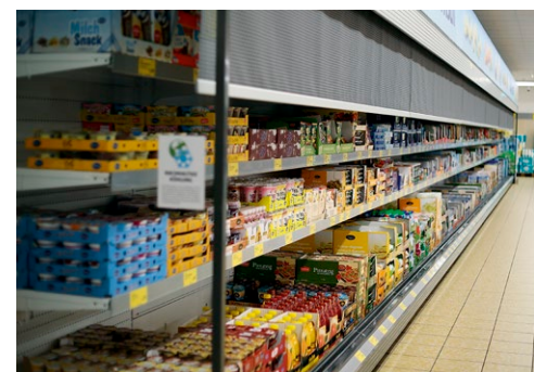
ALDI SÜD labels the cooling racks and cabinets which are operated with natural refrigerants with its logo 'Sustainable Cooling'
