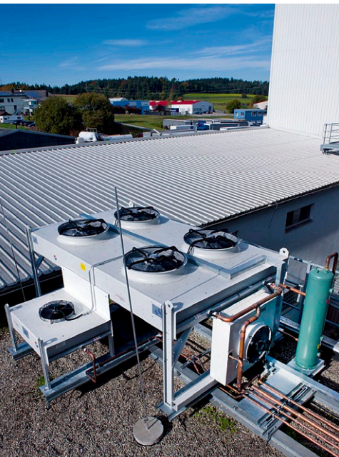
Condenser with an air cooled heat exchanger on the rooftop of the company
