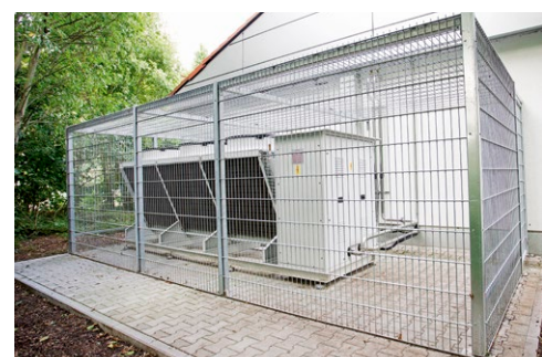
Right: The refrigeration plant at the back of the supermarket surrounded by fencing
