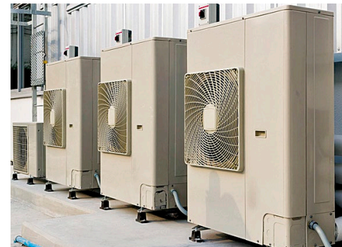
Refrigerators and air conditioners can contain climate-damaging fluorinated gases.
