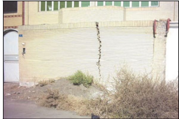
Figure. 6- Wall damages and unclosed features in Mashhad earth's surface
