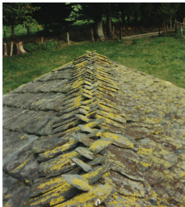
Figure 10 – Sloping roof made of crossed-slates called “cwerbas” in the Vielsalm area. Flanks of the slate roof are composed of thick purplish slates with various size called “cherbins”, Lierneux (Photo C. Legros).
