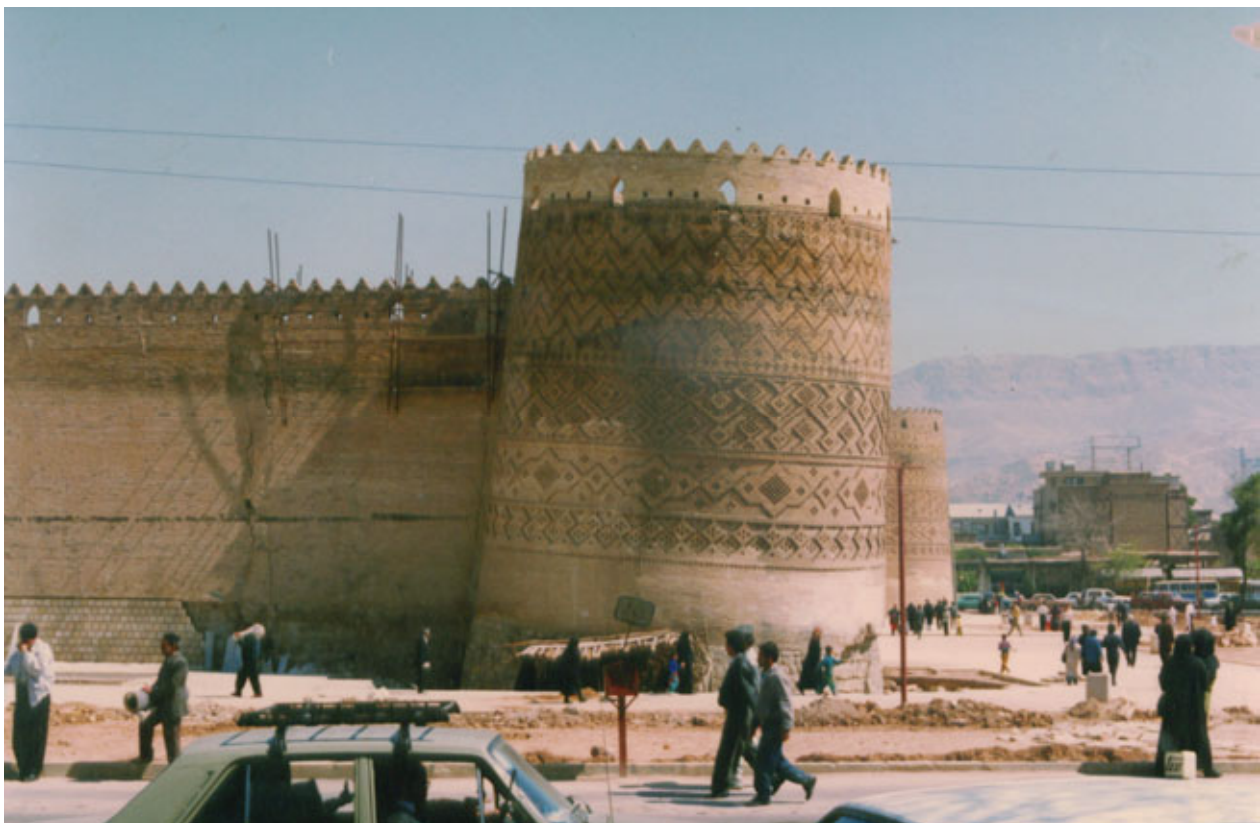
Figure 2- Deviation and damages to the tower and walls of Karimkhan Citadel in Shiraz (Rahnama-Rad, 1992).
