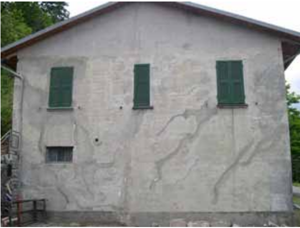
Figure 6 – Cracks in a house of Roccamurata.
