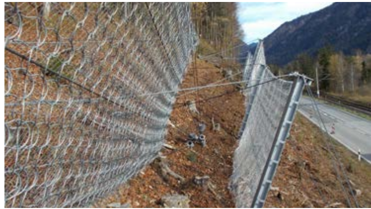
B 2, Rockfall protection fence between Eschenlohe and Oberau
