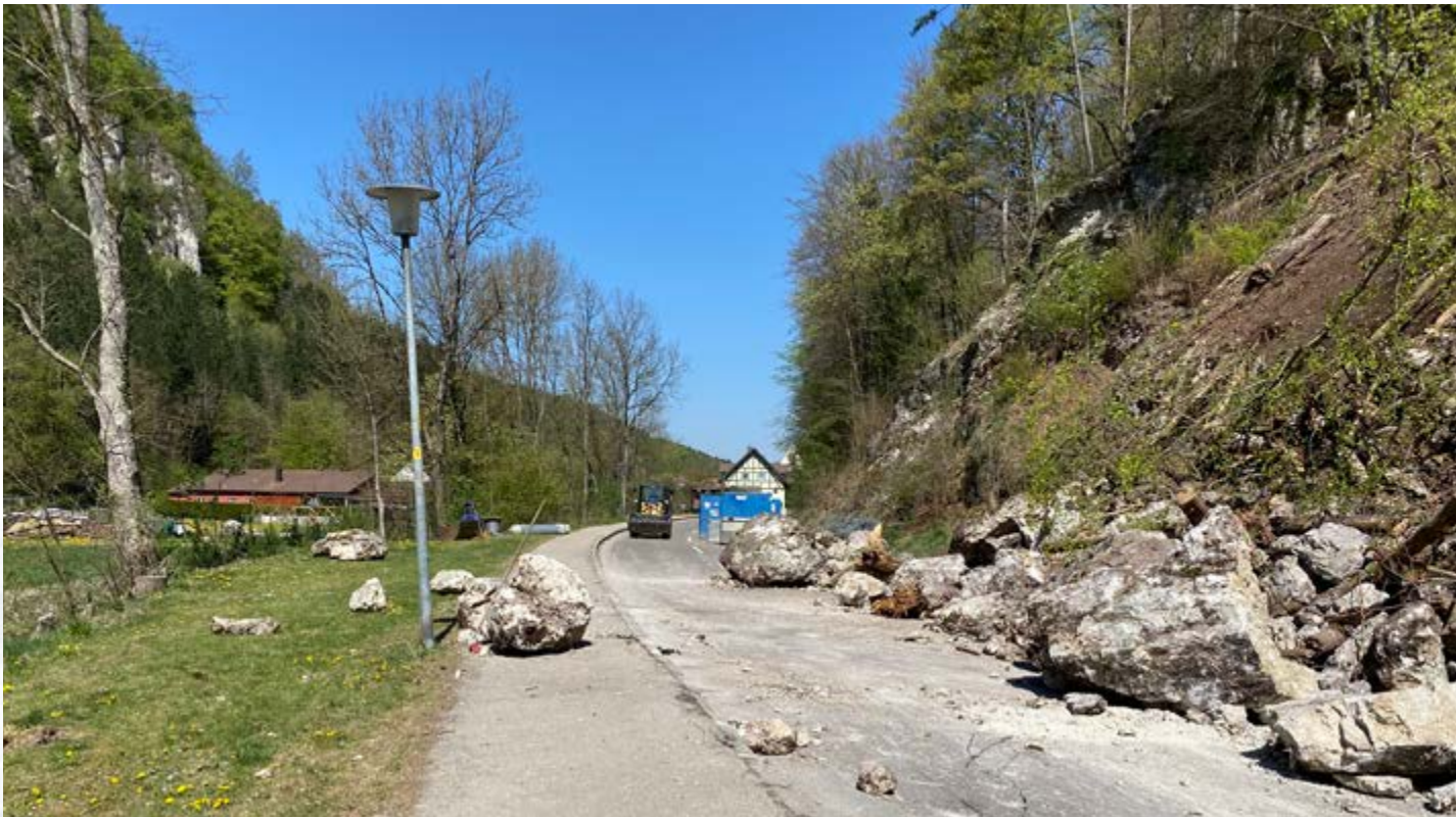
St2392, Rock clearance under full closure of the road at Kipfenberg in the Altmühltal valley
