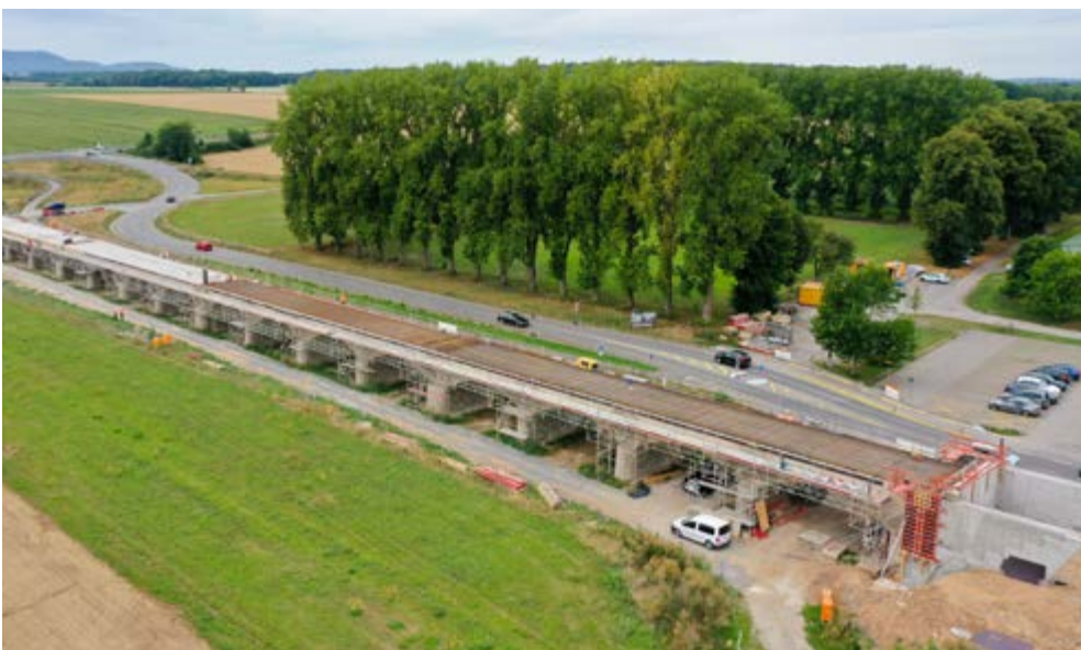
St 2275, Repair of the flood bridge on the River Main at Haßfurt
