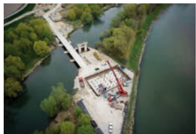
☞ St 2124, Plattling roundabout, new construction of the Isar bridge with lifting of the first steel parts at the abutment
