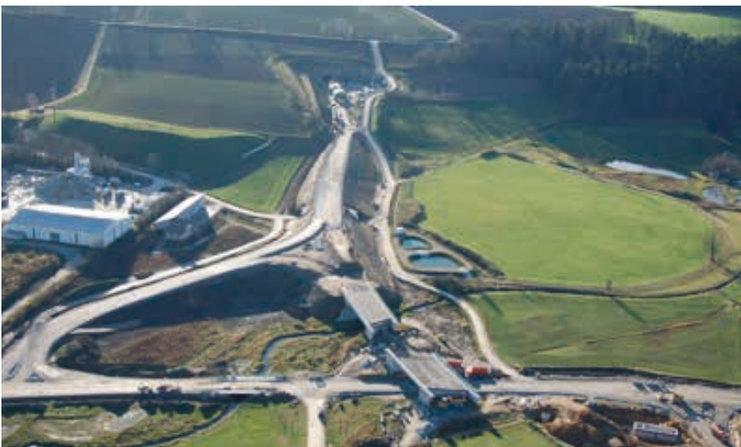
« B 20, Furth im Wald bypass, entry to the Deschlberg tunnel with Furth-Mitte interchange
